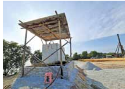
Proper basement for leakage control at diesel storage; E'Island Lake Haven
