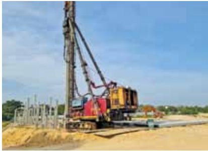
Drip plates below pile rig to prevent ground pollution at the E'Island Lake.
